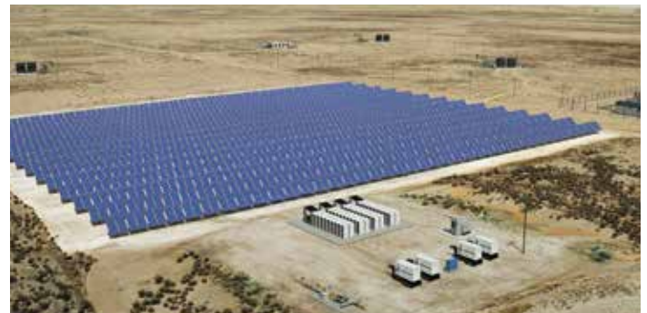
Array of solar panels, Baseline NexGen™ 400 mobile power generators, and storage batteries
